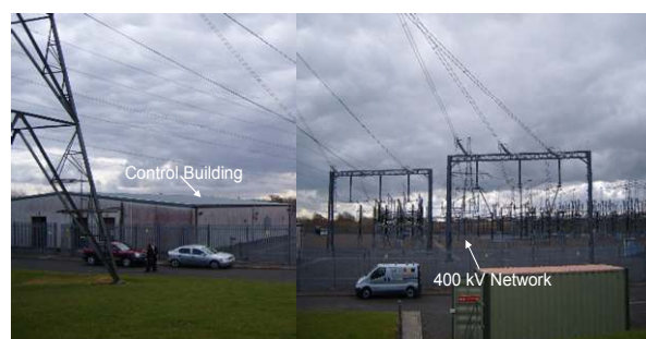
Fig. 3 Strathaven substation – 400 kV compound
