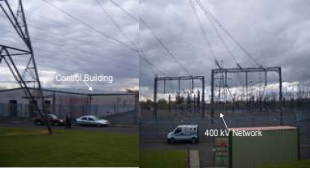
Figure 2 – Strathaven substation 400 kV compound.
